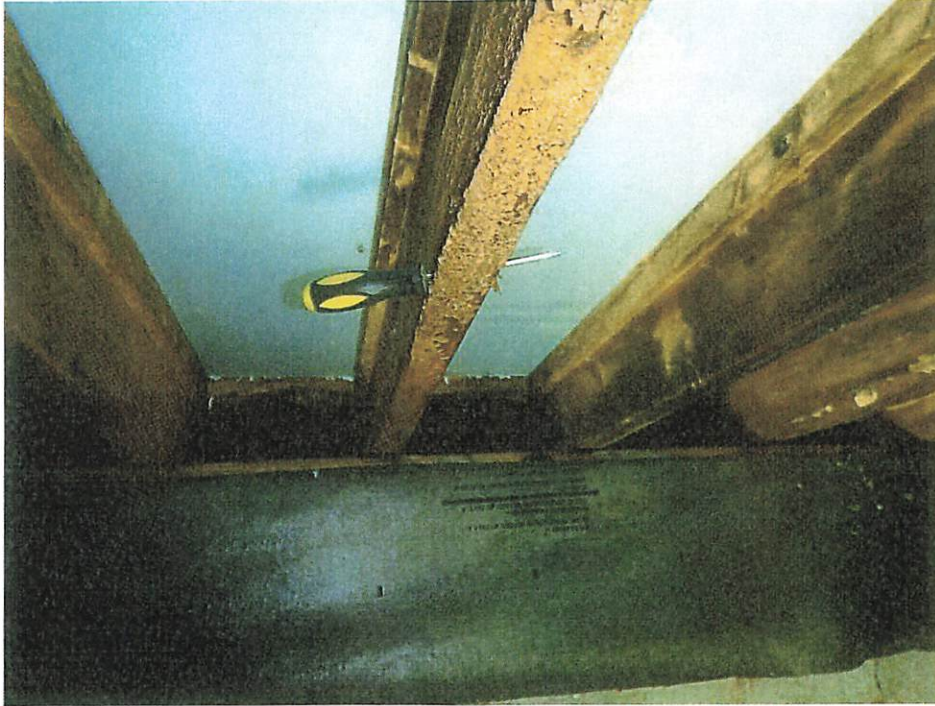
Photo 27. Photo illustrating extent of rot in addition floor joists
