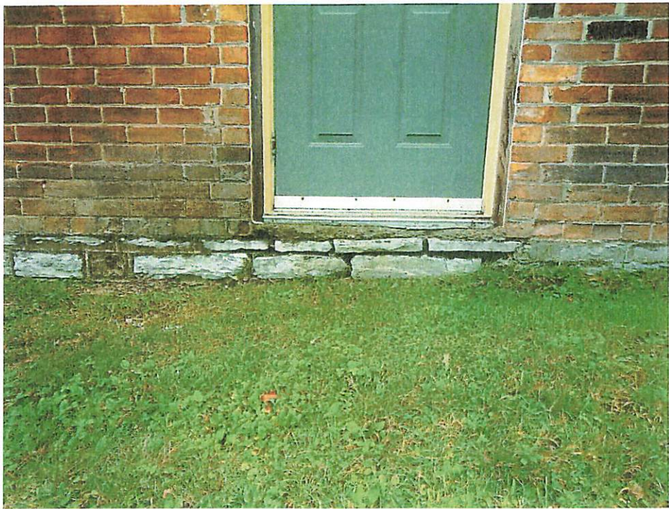
Photo 8. Mortar loss in exterior stacked stone foundation
