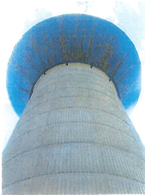
Residue and "growth" deposits under angled section
