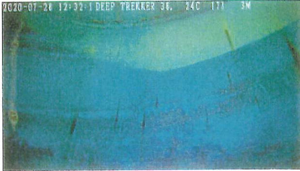
Wide view of tank wall random coating failures
