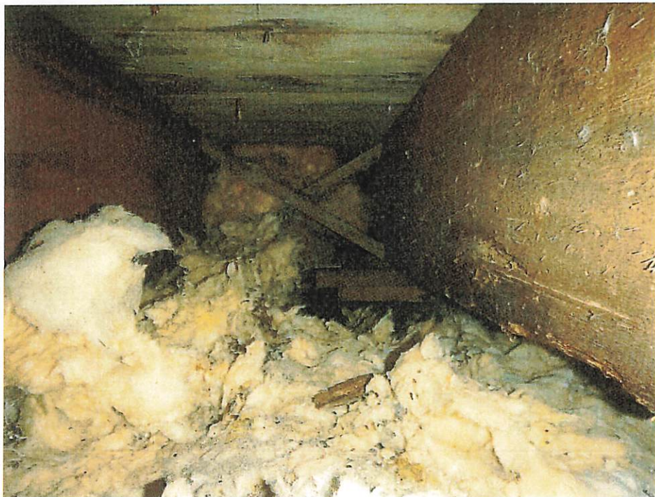
Photo 20. Damp batt insulation found in crawlspace under NW bathroom
