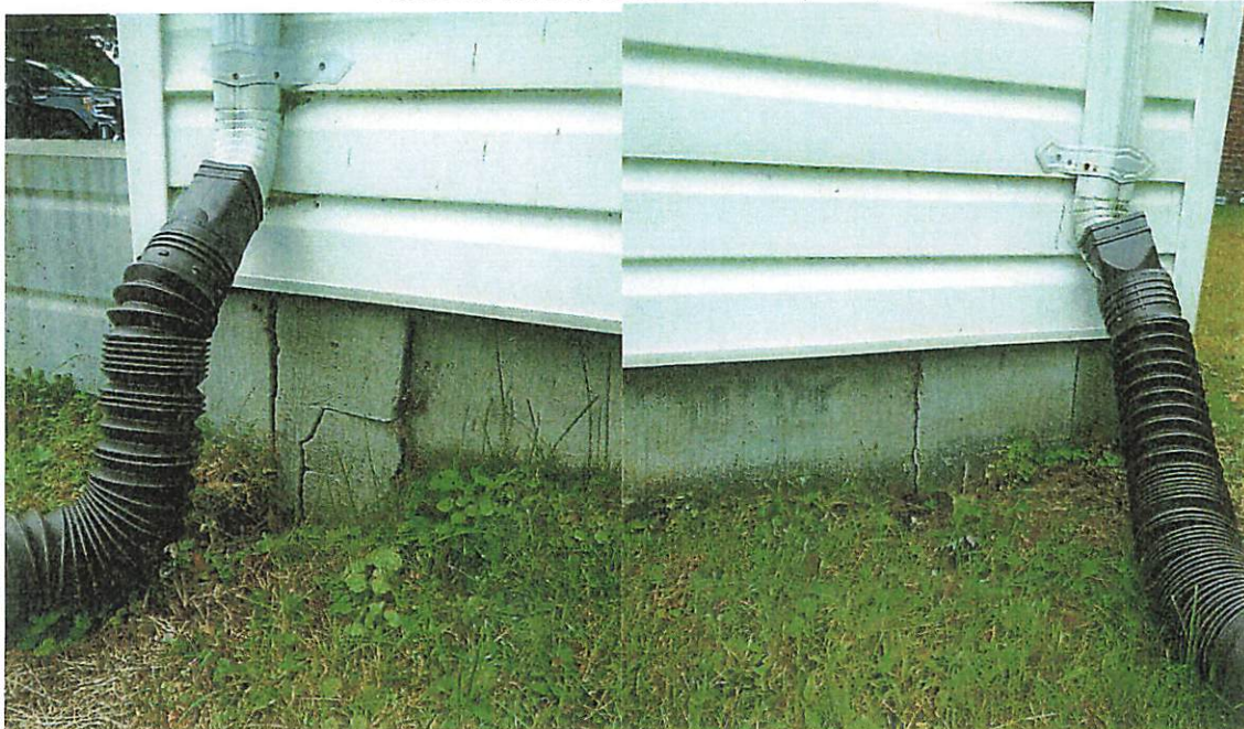
Photo 6a. Localized cracking in NW foundation
