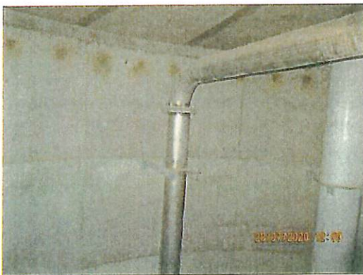
Overflow piping and inlet-outlet pipe section
