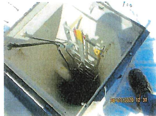
Dry riser hatchway open for roof access
