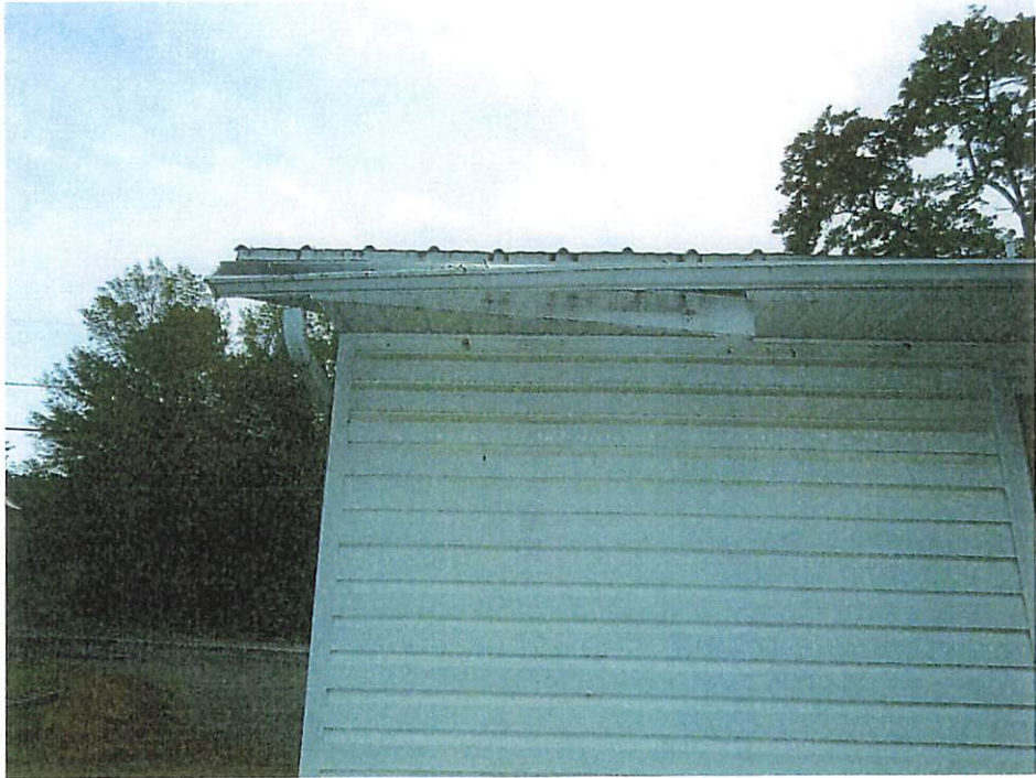
Photo 7. Damaged soffit in addition
