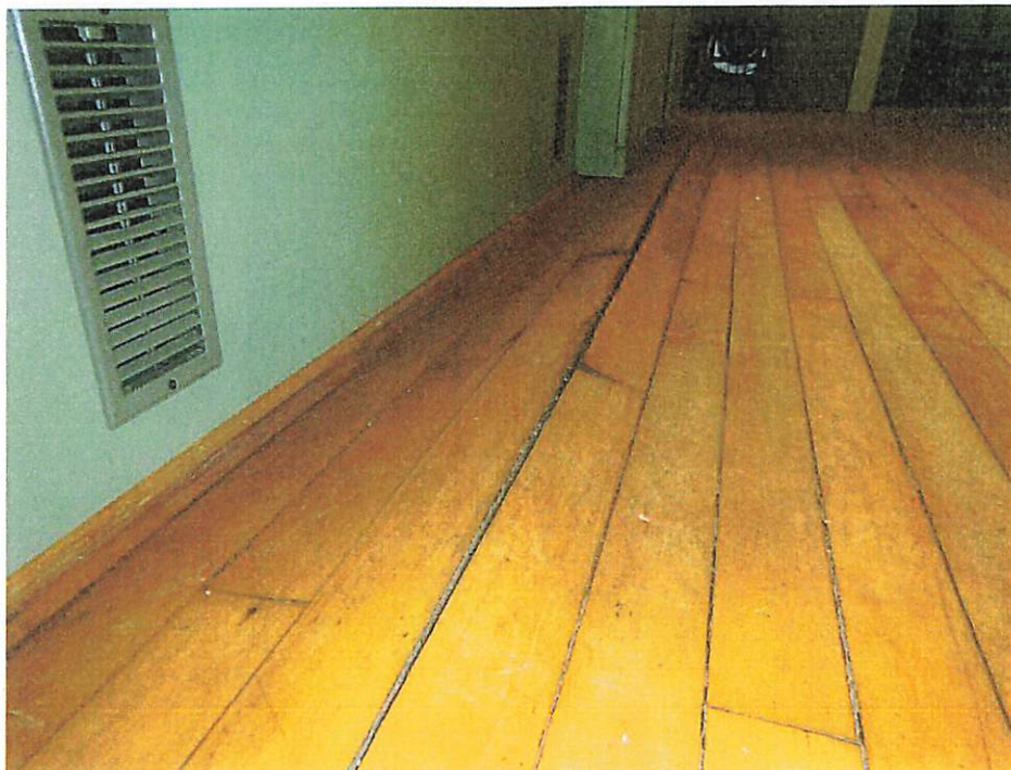
Photo 16. One location of heaved floorboards
