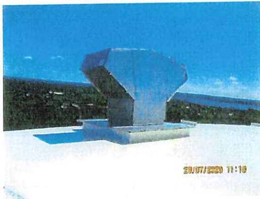
Roof top vent assembly in good condition
