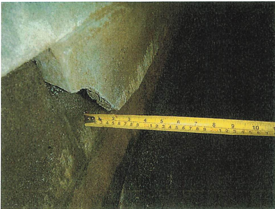
Photo 26. Photo illustrating 2" shift in addition foundation wall
