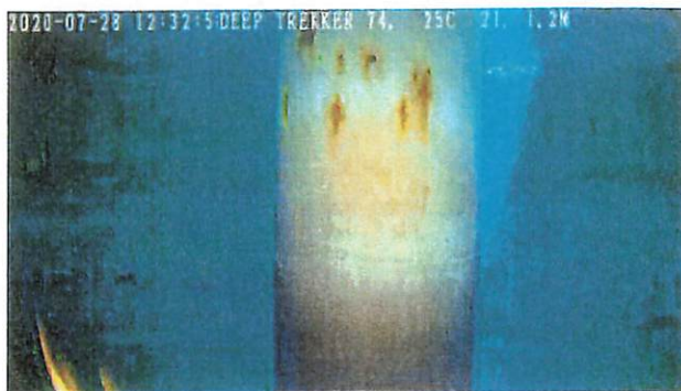
Areas of coating failure on upper areas of dry riser
