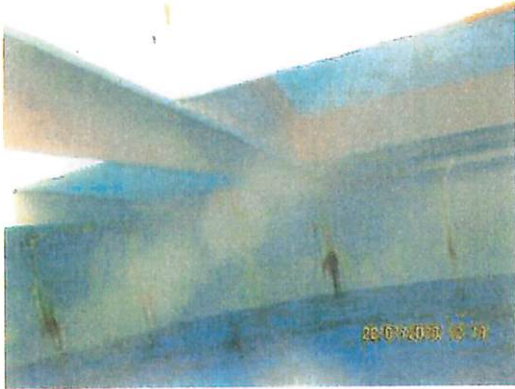
Typical internal wall view of coating failures
