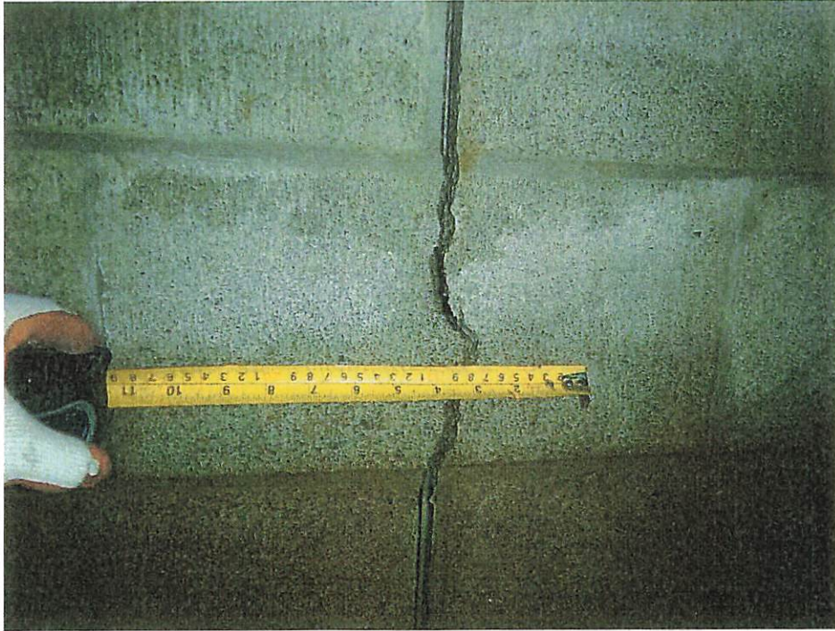
Photo 25. Wide crack in addition foundation wall
