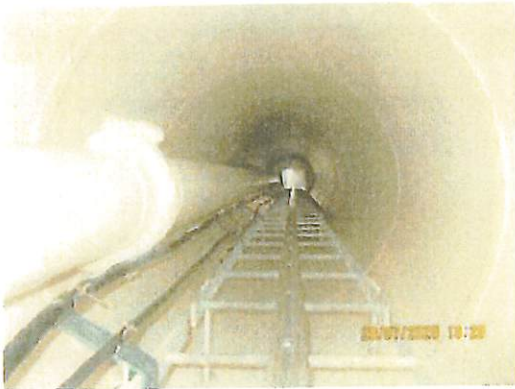
View directly up dry riser; roof hatch secured
