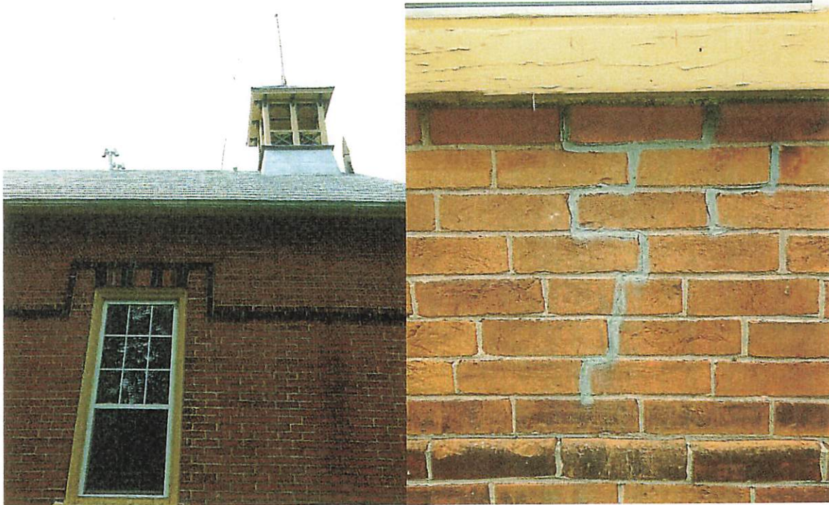
Photo 11. Localized step cracking in brick wall (several locations have been previously repaired)
